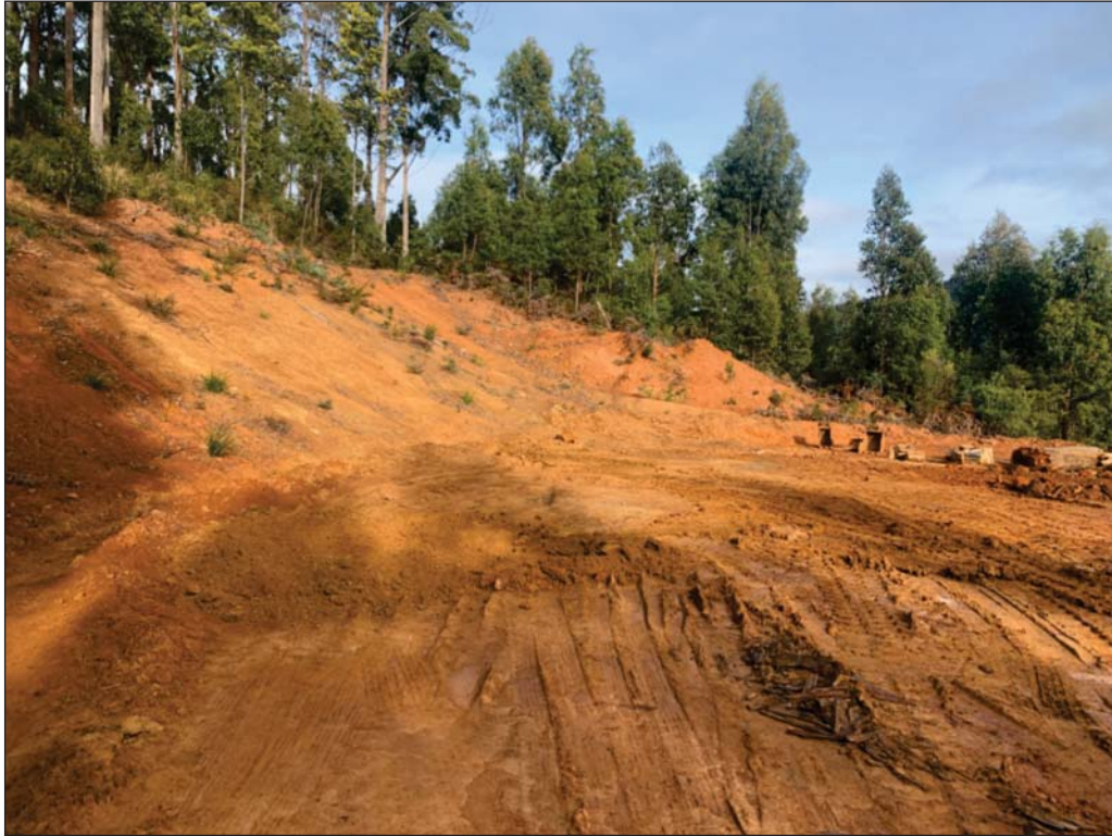
PLATE 1 - Looking southwest at the proposed building envelope and the cut batter above the site
